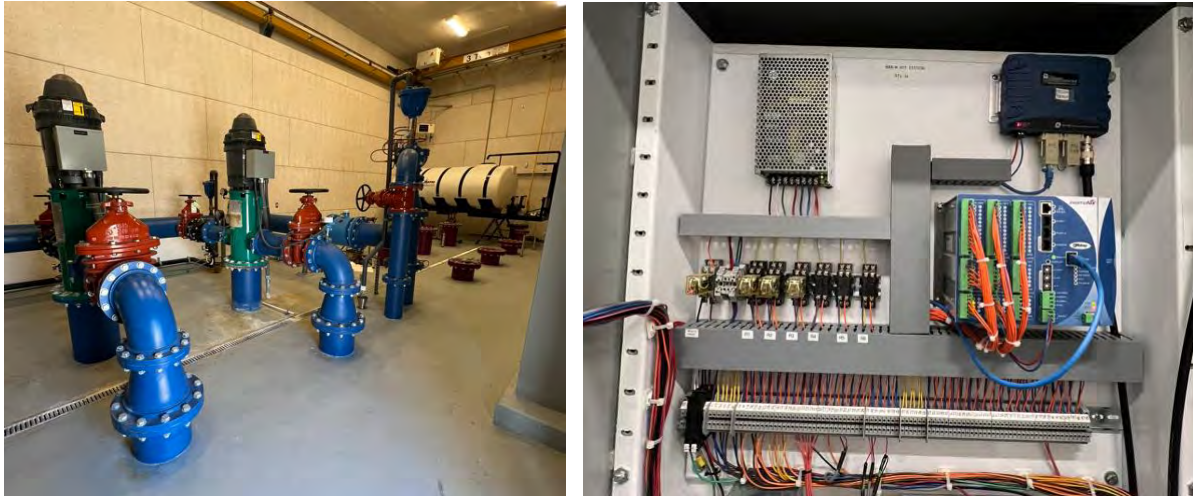
Figure A-19: 8000 West Booster Station
