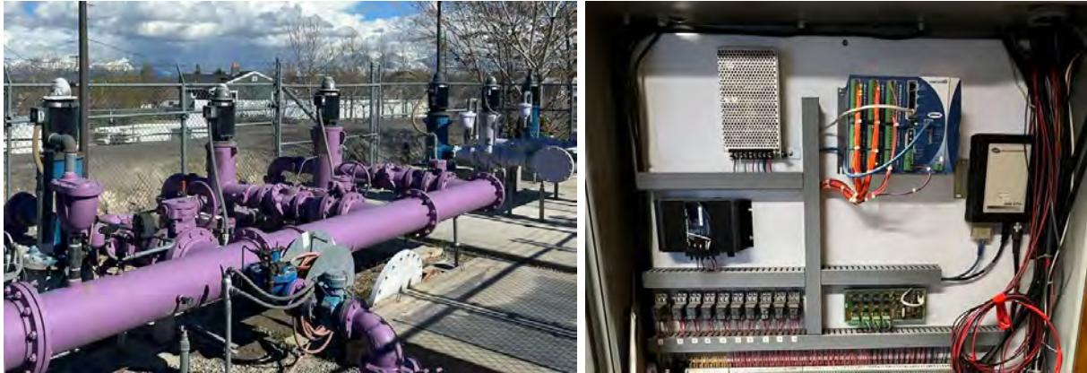
Figure A-21: Irrigation Booster Station
