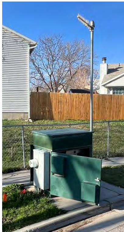
Figure 3-1: Lower Irrigation Well 2 Existing Control Panel Enclosure
