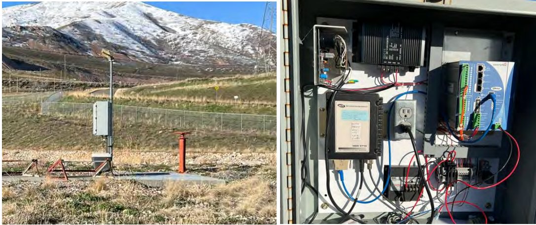
Figure A-17: Irrigation Zone 1 Pond
