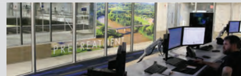
INSTRUMENTATION AND CONTROLS (SCADA)
