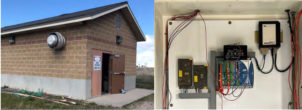
Figure A-6: Haynes Well 2 (RTU located at Haynes Booster Station)
