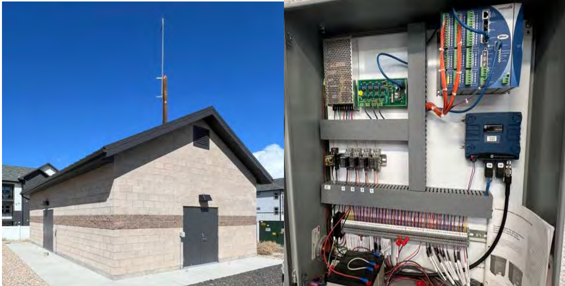
Figure A-22: Zone 3 Secondary Booster Station
