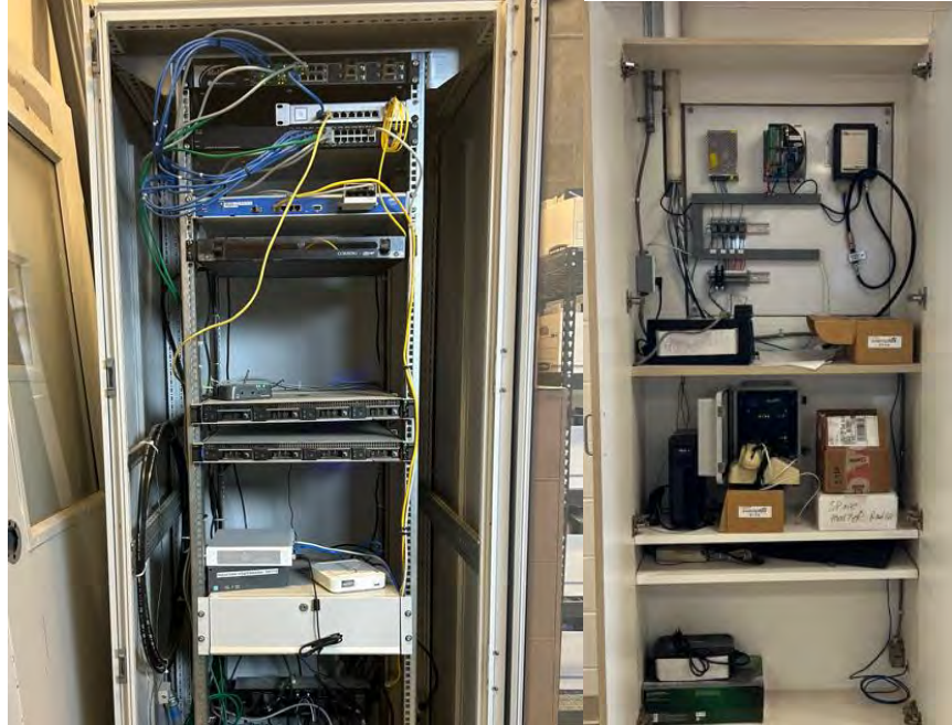
Figure A-25: EDR Water Treatment Plant
