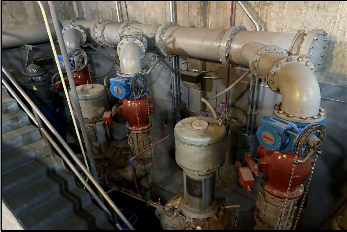
Photo 9 – Lower Level Pumps
