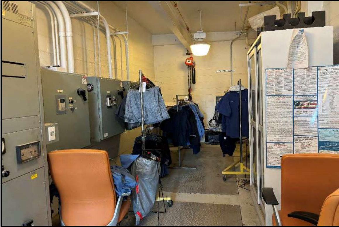
Photo 5 – Uniform Storage Area And Electrical Gear
