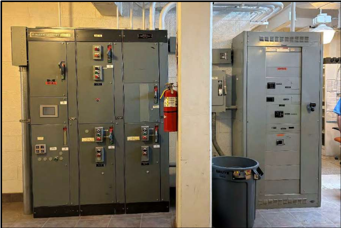
Photo 8 – Electrical Gear Outside Showers
