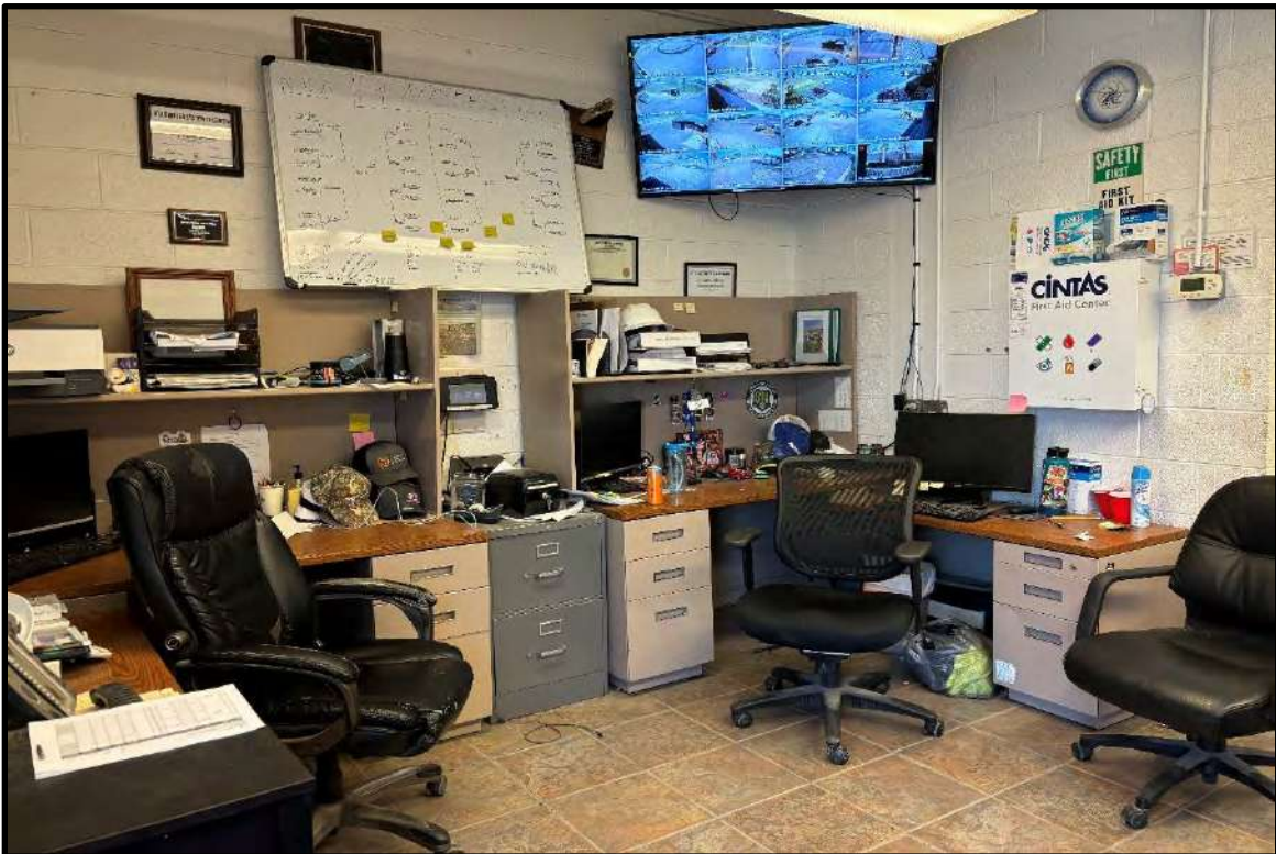
Photo 4 - Control Room/Operator Stations
